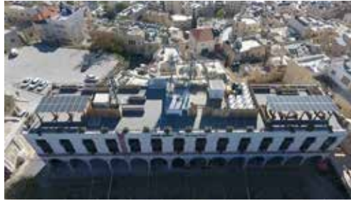
■ Mini-system and weather station on the roof of the engineering department of Bethlehem Municipality.
